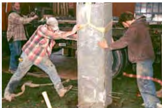
Setting the base with embedded rebar into hole and place 10 bags of cement around the base topped with topsoil
