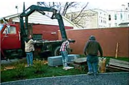
Jody Pod and sons Jody and Tator from Barnes Bluestone, install the base behind the renovated jail
